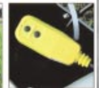
GFCI Plug-in attached
